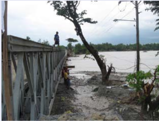
Bridge damaged by typhoons
